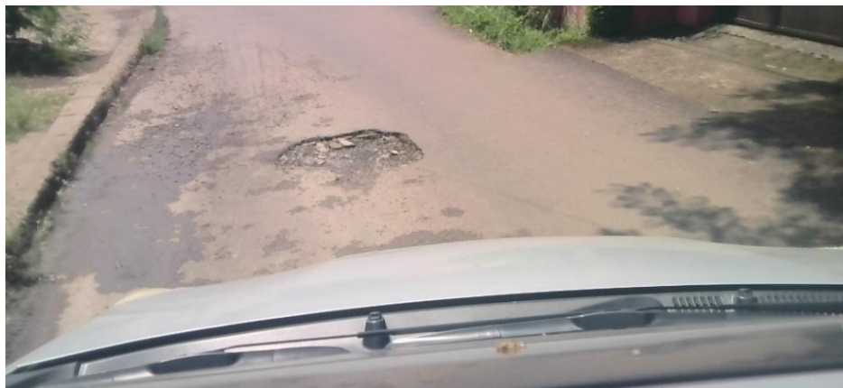
Figure 3. Example of Damaged Road Images in the Dataset
